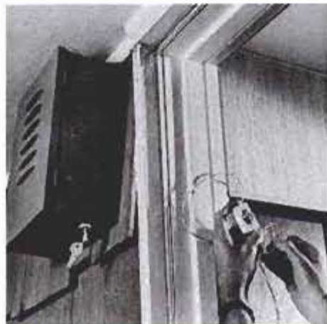
Test key and toggle switches and current in circuit wire. With either switch turned on, alarm should sound when wires are separated. If system is okay, turn switches off, mount toggle switch; then install and wire detectors at windows and doors.
