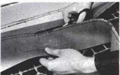
3 Press carpet firmly into floor-wall joint to transfer chalk marks, then cut.
