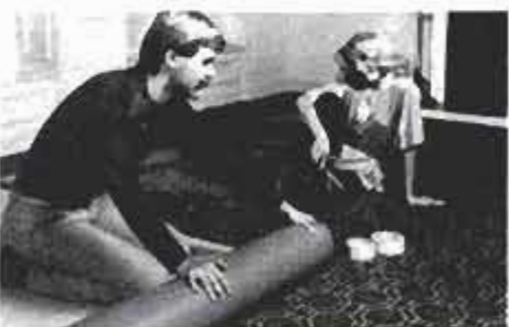
2 Roll the carpet onto the floor; allow a few inches of excess to run up the wall.
