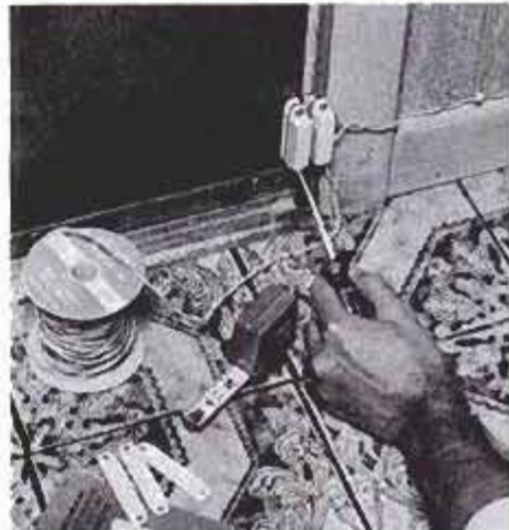
Attach unwired half of a magnetic detector to a door with screws. Often, surfaces are not flush, so use spacers available from Radio Shack. Cut and attach only one wire of the circuit line for each detector.
