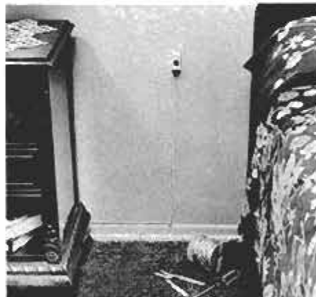
Panic switch is usually mounted close to the bed, but a perimeter system may have panic switches anywhere you choose. Since this switch is the last one in our circuit, ends of the two circuit wires are attached directly to the switch terminals.
