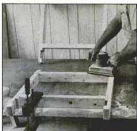
Assemble and finish-sand side pieces, then join them by adding the cross members.
