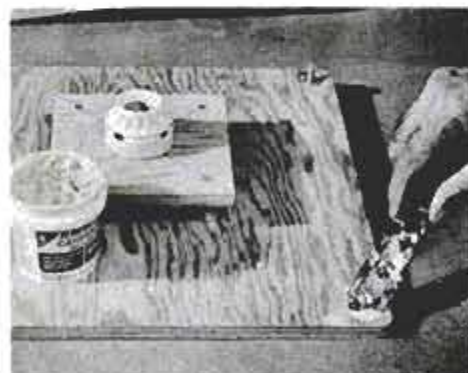
Rod Teenuts are recessed below surface and concealed with wood filler. Temporary screws keep filler from clogging threads.
