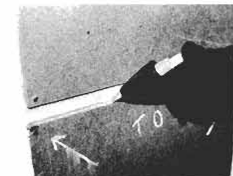
After all hardboard panels have been attached with screws, a hot adhesive sealant is applied with gun to seal edges.
