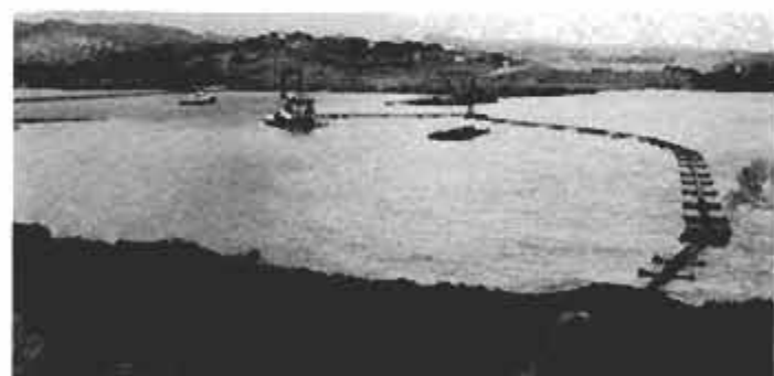
After this small bay is dredged, diked and filled with sand, the runway will traverse it. Miami-based dredging firm is the lone American contractor on project that showcases Cuban "friendship."
