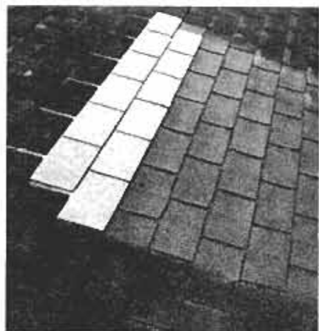
This test roof, shingled in 1967, has two rows of FRS (fungus resistant shingles) that stayed white. They also started to clean the mildewed shingles below them.
