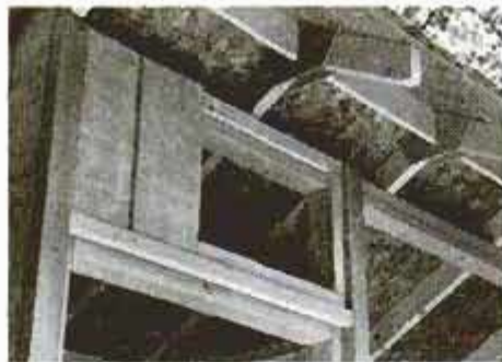
Area above door is furred out with 1 \times 2 strips before siding is applied. Cut small siding panels from any leftover scrap.
