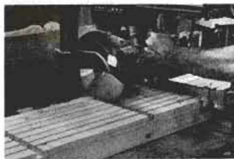
To make \frac{1}{4} \times \frac{1}{8} -in. shelf notches, clamp compartment studs together and make several kerf cuts. It's 4\frac{1}{8} in. between stud bottom and lower notch and 5\frac{1}{8} in. between stud bottom and upper notch.
