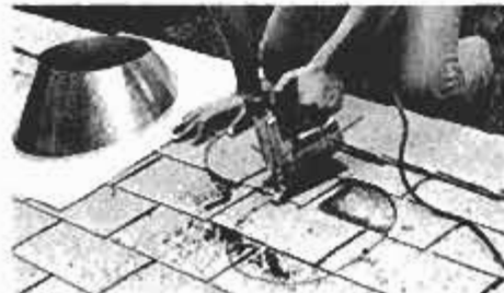
Cut a hole through the roof for the chimney with a sabre saw. Use the same method for determining center point on the interior side of the roof as used on the ceiling. Bore a hole through center point.
