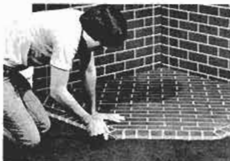
Cut the carpet with a mat knife, using the floor panel as a template. Abut floor panel against temporarily placed wall panels.
