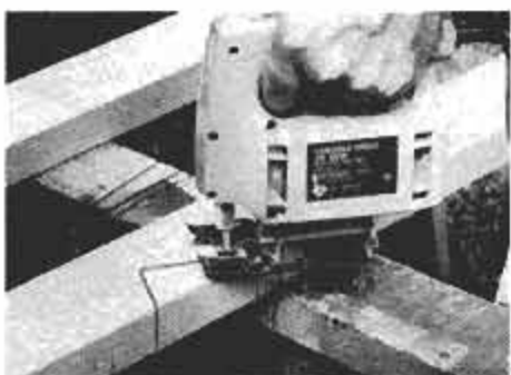
Use sabre saw to cut rafters. When pattern is complete, use as template for others.
