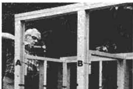
Frame front and back walls, then sides. Toenail stud bottoms to floor and tops through plate as shown. Blocks (A, B) give nailing surface without using whole stud.
