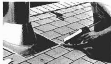
Run a bead of silicone sealant along side edges of flashing after it is nailed to roof. Before nailing, sealant was applied under upper edge and both sides of flashing. Lower side is not nailed or sealed.
