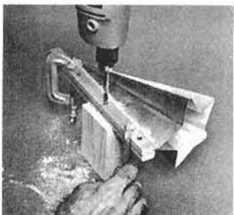
6 Clamp wood strips to metal flanges; bore the holes, ending with \frac{3}{16} -in. bit.
