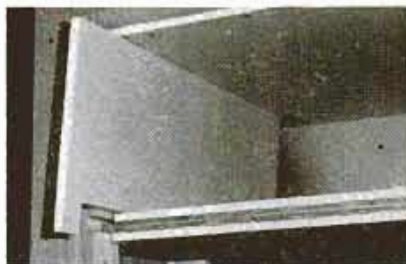
With ceiling, shelf assemblies and back walls installed, cut upper sides to fit. Small tail in front covers notch in front studs.
