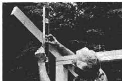
Rafter pattern is made by tacking board to top plate end. Mark position for bird's mouth cuts, then use level to make plumb cutoff lines for ridge and rear overhang.
