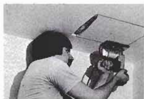
Cut a 14½-in. square out of the ceiling with a sabre saw. Bore a pilot hole in one corner of square to insert saw blade.
