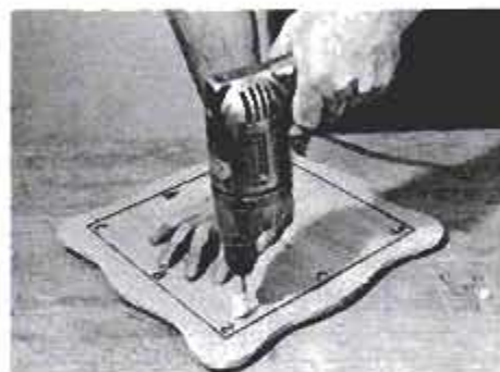
32 Bore holes 1/2-in. deep using masking tape as a gauge. With accurate transfer, real top should fit as neatly as false one.
