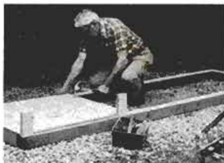
After base is assembled and leveled, nail on compartment floor using 8d galvanized nails. Use scrap stud blocks to keep plywood 1\frac{1}{2} in. back from front edge.
