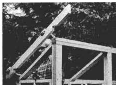
Rafter is ready for nailing. Drive one nail through top of both notches, into plates.
