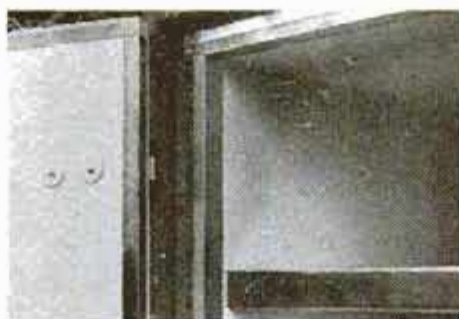
View shows completed metal-edging job. Fender washers and hinge bolts on door will clear jamb when door is closed.
