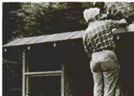
Cedar shingles are applied over a layer of 15-lb. felt. A 5\frac{1}{2} -in. exposure to weather was used on front and 7\frac{1}{2} in. on back.
