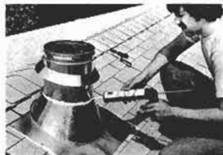
Apply sealant between the top perimeter of the flashing and the chimney. Collar is then lowered and more sealant is applied.
