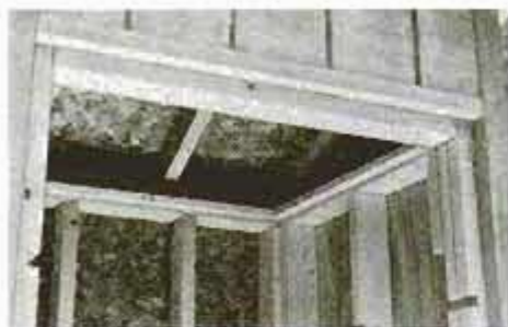
Furring is nailed to sides and back top plates to receive drywall ceiling. Bottoms of strips are at same height as door header.
