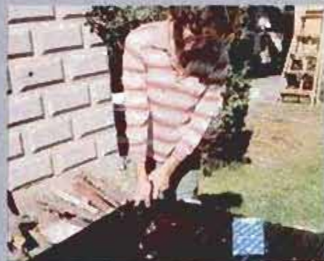
10 When splicing sections together, seal the seam with silicone caulk; then secure with Pop rivets. Before installation, seal top and bottom edges with adhesive foam.
