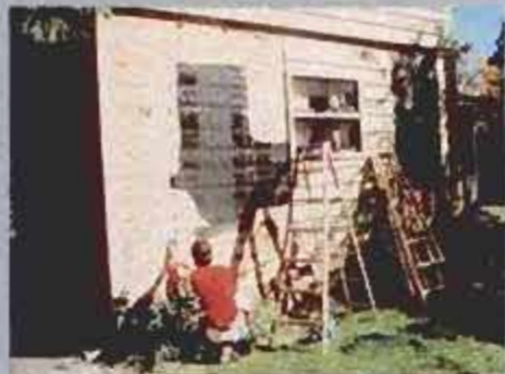
2 Remove siding (centered over a stud) to accommodate TAP frame and support.
