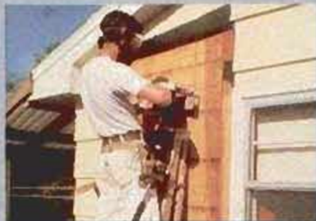
3 Cut upper and lower vent openings in adjacent stud cavities at the extremes inside the TAP frame; finish cuts indoors.
