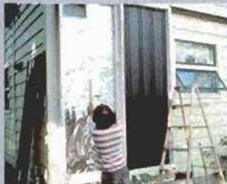
11 Glue and nail a nailer centered on the Thermoply; weatherstrip the absorber plate sides; attach it to the nailer and frame.
