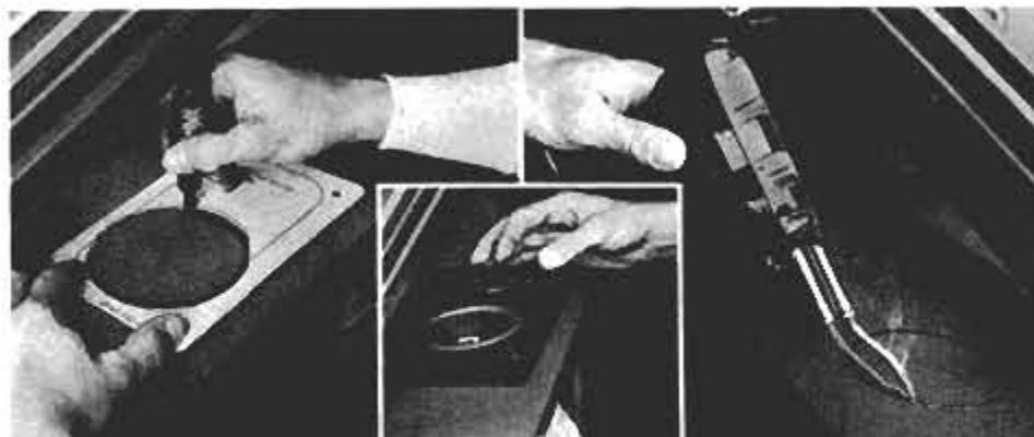
EPI model LS-70 speakers in rear could mount flush or on top of trimwall. We used template supplied to mark out mounting hole for an on-top installation (inset).
