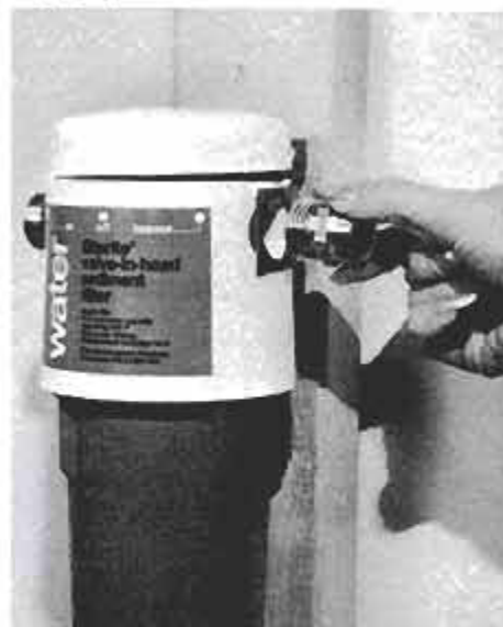
A male-threaded pipe fitting holds the filter securely in its bracket. The adapter allows you to hook up the filter to the existing piping in the cold-water line.
