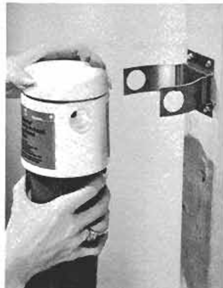
This sediment filter is installed on the main cold-water line. The pipe openings in the filter head line up with bracket holes.
