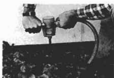
Space soil injections 12 in. apart and 6 in. from foundation around house perimeter.
