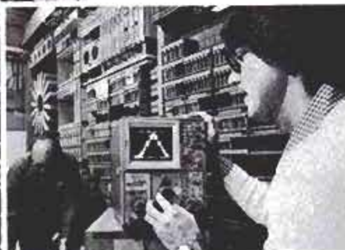
The master switching complex is the heart of the AMPS system. Here, a computer will decide how a message is to be routed.
