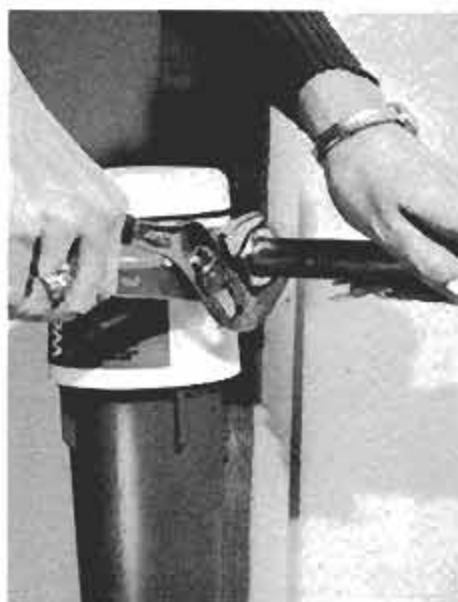
Tighten the nut firmly, but not excessively. This in-line filter has a water bypass valve to facilitate any cartridge changes.
