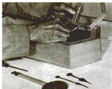
Carefully hinge the access door so it doesn't bind when it closes. Hinges are mortised into both door and the frame.
