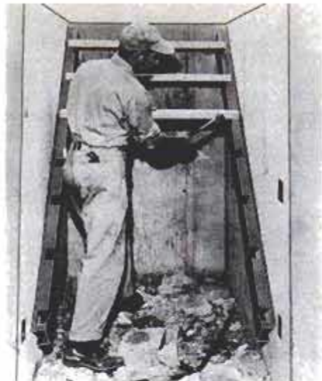
Stair stringers are attached to areaway walls with masonry nails. Install treads.
