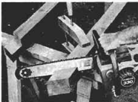
Clamp post firmly to sawhorse; keep saw level when making mitered shoulder cut.
