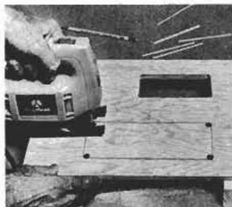
Bore holes in the corners, then use your sabre saw to cut out the window openings.
