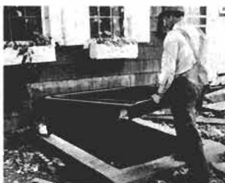
Adjustments are made before the door is attached. Here, header slips under siding.
