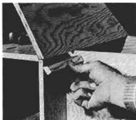
Strip (K) is added to extend overhang after through bevel cut is made on bottom of roof panel. Piece is then glued and nailed.
