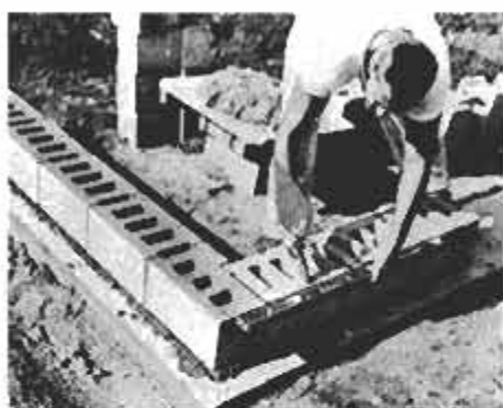
After three or four blocks have been laid, corner block is used for correct alignment.
