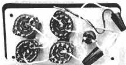
Wire the rotary and pushbutton switches. Use solderless connectors to connect the switches to the garage-door opener.
