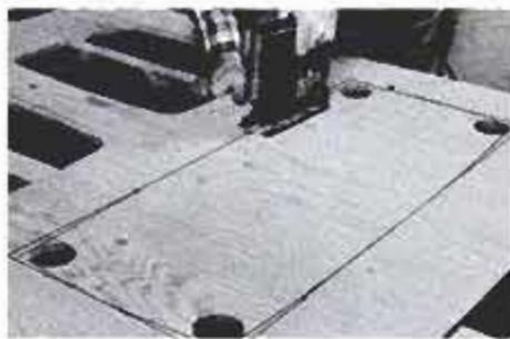
Holes made with a 2-in. hole saw form corners of the cutouts. If made with a portable drill, be sure you clamp workpiece.
