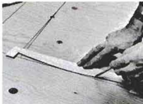
Thin cardboard templates simplify the layout of the cutting lines for the openings.
