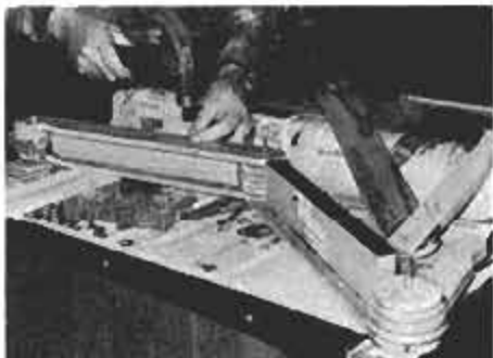
Boom and arm are assembled with axles and sheaves in place temporarily for fit.
