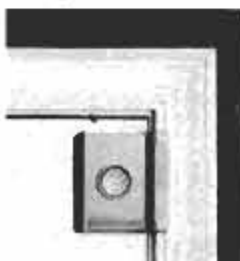
This photo shows a transmitter & magnet installed. If a break-in attempt occurs, separating the two, the transmitter sends a signal to the console which sounds an alarm to scare away the burglar. Installation takes only a few moments & doesn't even require a screwdriver.
