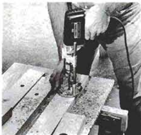
If you must bore the holes with a portable drill, a drill guide is invaluable. Bore the larger holes on outside members first.
