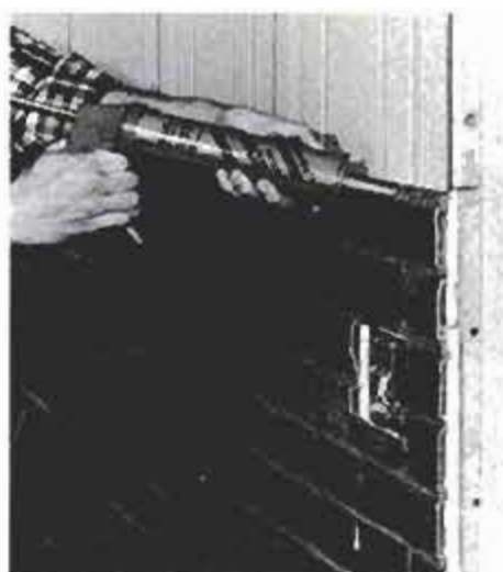
Mortarlike joint material adds finishing touch to the fireplace wall. The mortar and keystone arch give an authentic appearance to the imitation-brick panels.
