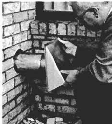
A hole is cut to the outside just below floor level and the wall cap is installed. The cap contains a damper to prevent backdrafts when the grill is not in use.
