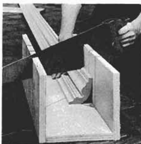
Urethane-foam reproduction of an 18th-century molding can be tooled as if it were made of soft pine. First prime it; then cut it in an oversize miterbox as shown. Similar molding is used for the baseboard, the casings, on niche surround, and on the mantel that's in the office.
