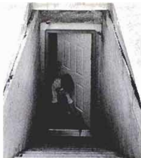
A cartridge-actuated hammer is helpful in fastening the threshold to the concrete floor. A steel door secures the exterior entrance. Stairway comes preassembled.
