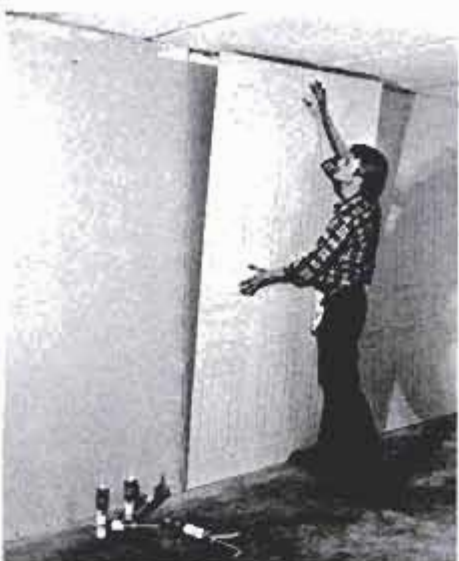
After drywall was applied over the insulation, paneling adhesive was used to secure the paneling. The deep etching on the panels adds to the room's traditional styling.
