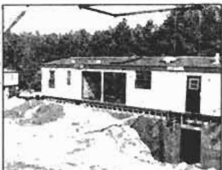
Factory-built house is lowered onto the foundation, which must be accurately built according to homebuilders' plan.
