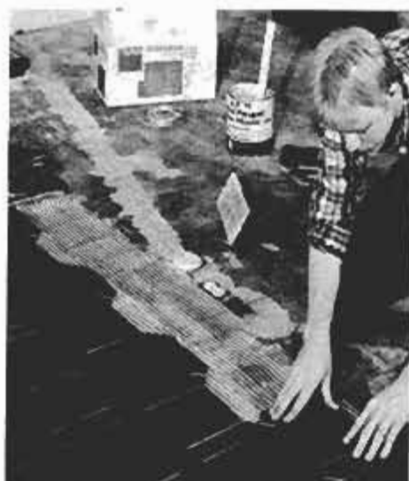
Oak parquet floor tile is laid to complete the home office. Electrical outlets, a phone jack and an additional conduit for future power additions to the home office are visible.
