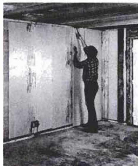
Insulation \frac{3}{4} -in. thick is glued to the wall between top and bottom furring strips of same thickness. A 2x4 is temporarily nailed to strips until the glue sets.
