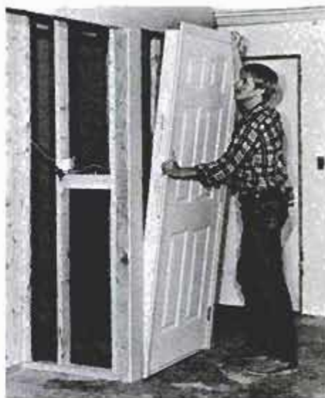
Factory-made door comes prehung in jamb. Latter slips into rough opening and is shimmed and nailed in place. This saves hours and makes the job an easy one.
