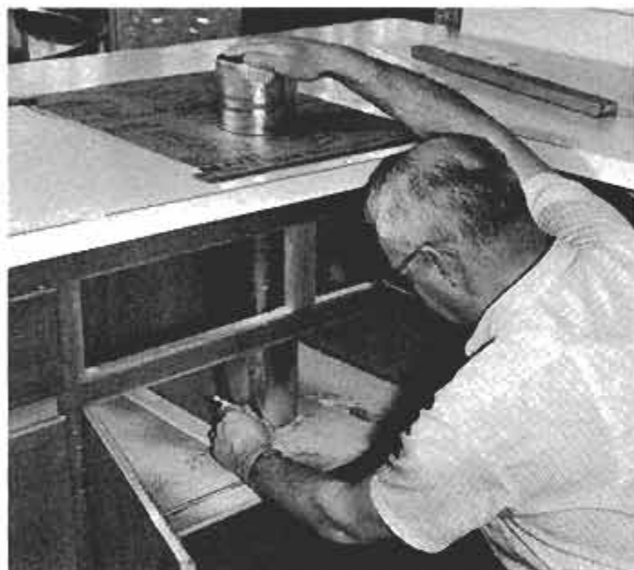
After you have cut countertop, use same template to mark the location of the smoke-vent ductwork. By lining up the duct carefully now, attaching the two will be much easier later.
