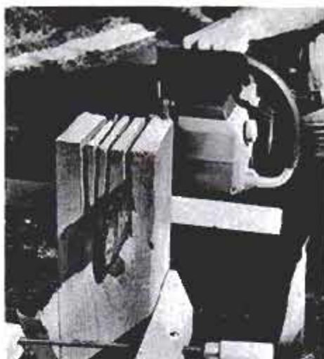
Make four or five kerf cuts to notch out the post top. A length of wood across the back is the depth guide for each cut.
