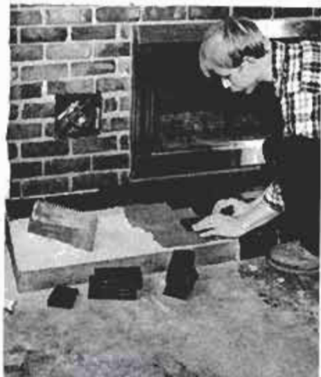
For a good-looking, low-maintenance finish, glazed ceramic tile was applied to the hearth. Grout that matches the mortar lines of the adjoining brick is applied later.
