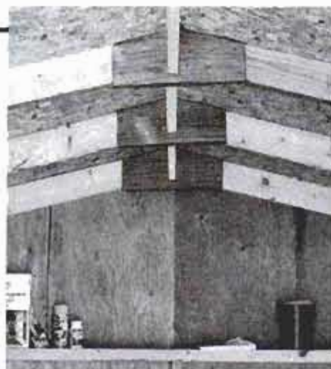
Because structure lacks collar beams, roof is beefed up with gussets over all joints.
