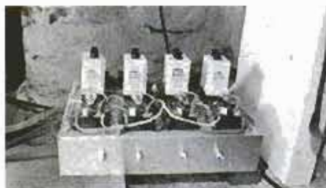
Four voltage-sensitive relays kick on in sequence to add load to Langhorne's system when power supply exceeds demand.
