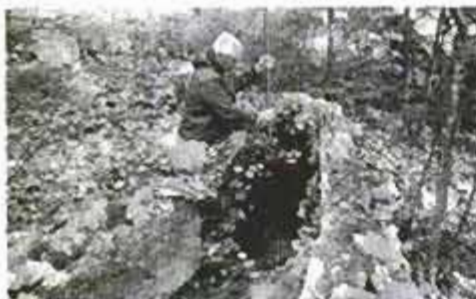
Mountain stream is diverted to enter supply pipe, lined with polyethylene. Screen keeps out leaves, sticks and debris.
