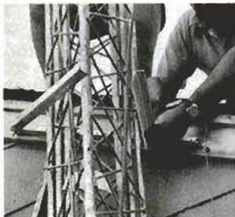
House bracket is lag-bolted to rafters in the roof and located close to the tower.
