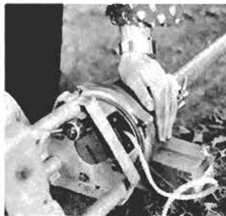
Rotator is attached to the plate on top of the tower. Note that the control cable is connected before the tower is raised.
