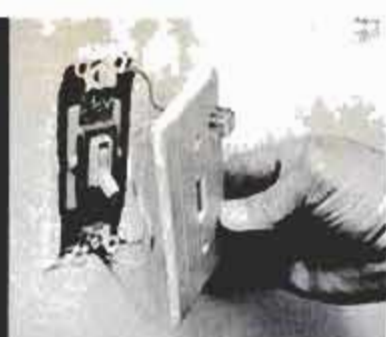
After installing the indicator, test the lamp to be sure that it is connected correctly before you reinstall the switch plate.
