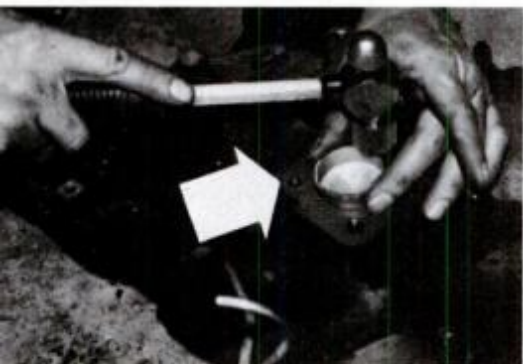
Freeze plug (arrow) is hammered into the intake manifold to block air/fuel flow.
