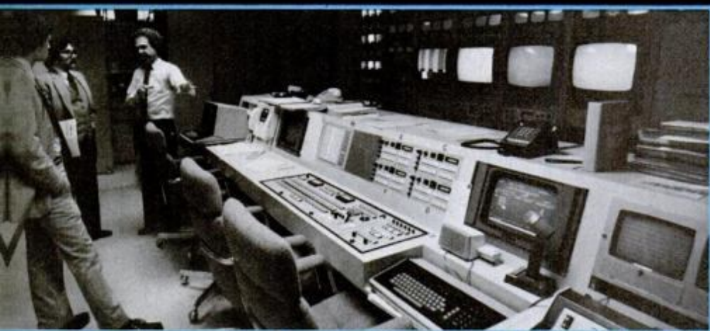
Movie channel's main console (shown: Home Box Office) monitors signals to satellite.
