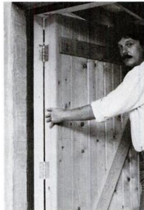
Thick doors with Styrofoam core help hold heat in basement. In addition, 4-inch-thick Styrofoam plugs block off basement windows to bottle up energy from greenhouse.
