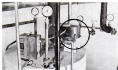
Problems did arise with pump (circle), and the manufacturer replaced it at no cost.
