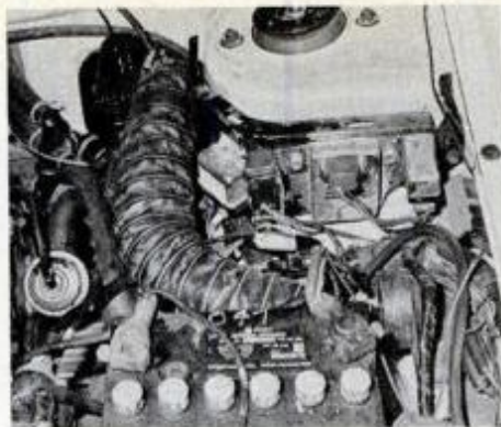
From left are antideseling relay, starter relay, voltage regulator and radiator-fan relay (on airconditioned cars).
