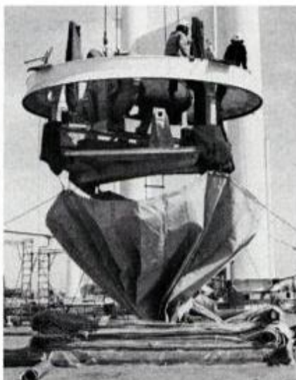
Hoist lifts tent from center ring. Once out of crate, the bottom edges are pulled outward like an umbrella.
