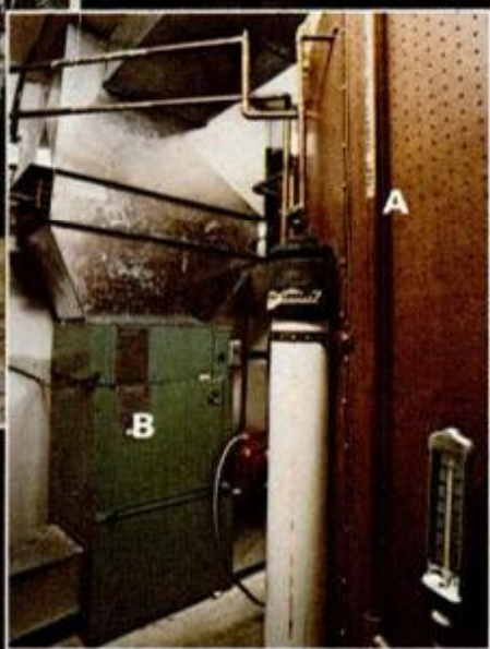
Panelized storage tank (A), capable of storing 1.5 million B.T.U.s, is well-insulated and made with a heavy vinyl liner. Air-handling unit (B) transfers heat from water to air and distributes it throughout the house.
