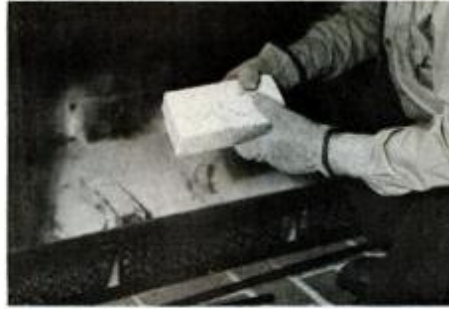
Place firebrick on edge to support logs. Cast andirons are costly and breakable, but firebrick is cheap and permanent.
