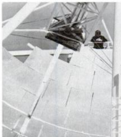
The boiler moves above 430 mirrors.
