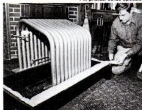
Fiberglass insulation, which comes with the unit, goes in next. Notice that the log retainers and leveling legs are installed on the unit at this stage of assembly.
