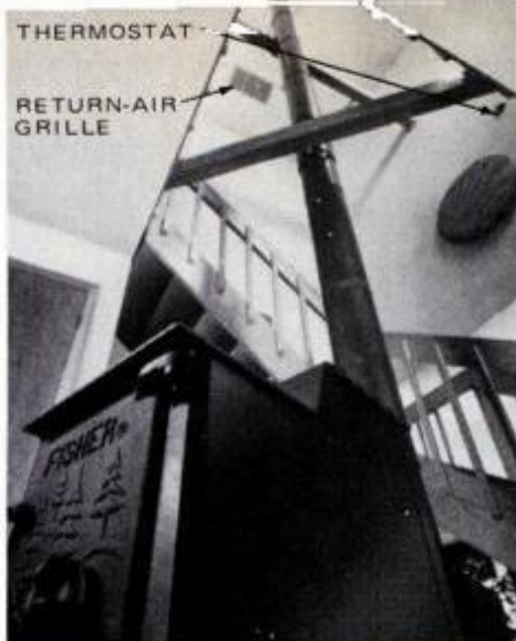
Air, warmed by stove, rises via stairwell and then is recirculated throughout house.
