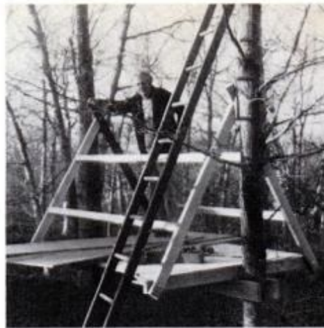
The floor is framed and skinned to provide a safe working platform so that the work on the A-roof can proceed.
