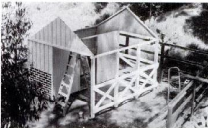
The barn is built of preassembled panels, small enough to be constructed in a garage or shop during the winter months.
