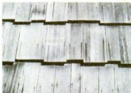
Nongalvanized or poorly galvanized nails will rust and stain siding. Eventually, disintegrating nailheads will lose holding power, causing the shingles to loosen.
