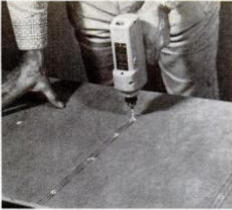
Bore lead holes for following nails along the center of all butt-joint locations. This is done to make certain that the nails will center in the mating pieces.
