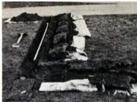
Check out system above ground for leaks and coverage. Then bury lines in V-shape trenches 8 in. deep. Replace sod, tamp.
