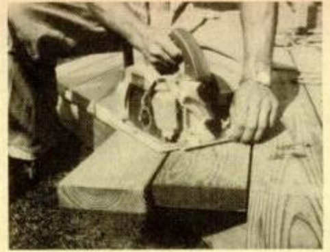
The 2x6 decking is installed with waste overhanging header. When all is down, a chalkline is snapped, decking is trimmed neatly using a portable circular saw.
