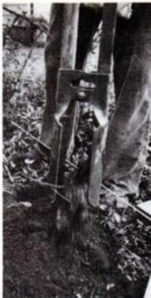
Each scoop removes a good amount of soil. Deposit it nearby for easy backfilling.
