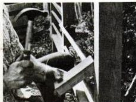
Cut 1x6s slightly full to gain a force fit; tap board in using a block of scrap wood.
