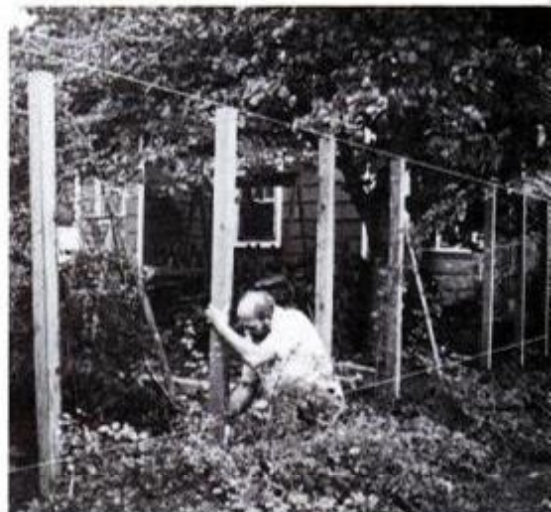
Posts can be cut before planting and set to touch elevation line, as here.
