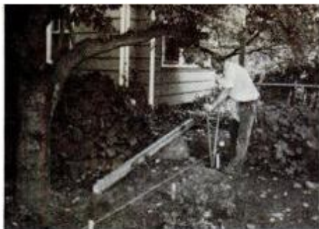
Fence route is marked using stakes and mason's line. End postholes are dug first.
