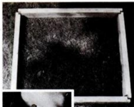
The gate frame, constructed of 2x4s, is rabbet-joined at the corners and is glued up with two-part, waterproof resorcinol glue.
