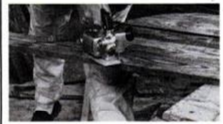
After constructing gate, use a sabre saw to cut the top to the desired shape.
