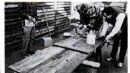
Gate is assembled by butting 1x6s; the brace nails are driven at an angle.
