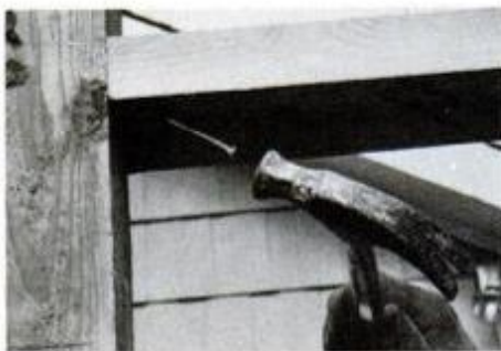
Second rail is toenailed to posts at both ends, and spiked to the center post.
