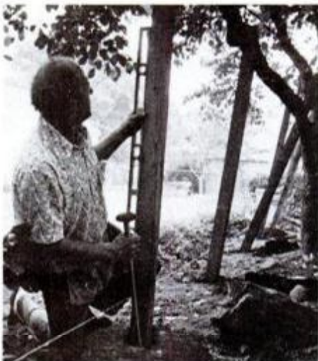
Use a spirit level—in both vertical planes—to make certain post is plumb.
