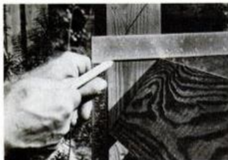
Louver installation starts at bottom; a square aids placement of next board.
