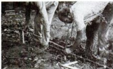
Stakes are driven along the line at each point where an intermediate post will go.
