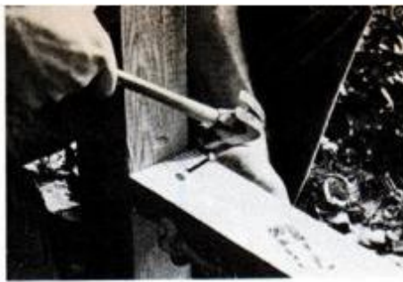
Horizontal rails are fastened using 10d common nails toenailed at joint with post.
