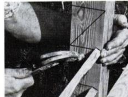
Nails are toed through louver face; dull points first to prevent any splitting.
