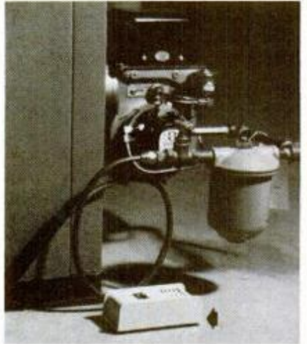
Alarm, placed at base of furnace, will sound if basement floor becomes wet.
