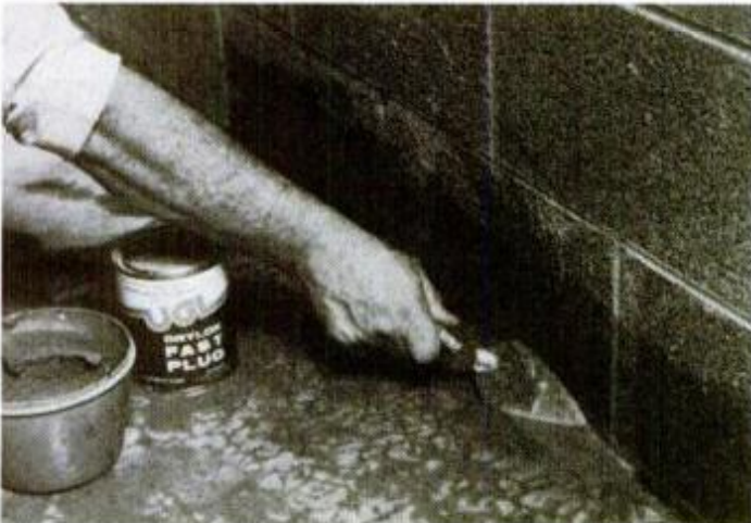
Before applying sealer, use wire brush to remove loose debris; then plug all holes and floor/wall seams with patching mix.
