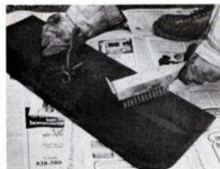
After removing damper, scrub with wire brush. Then clean smoke-rise box, using flue brush with one or two rods.
