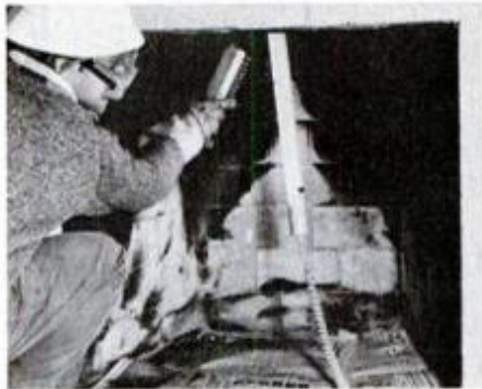
Clean creosote accumulations from fire-box walls with a hand wire brush. Trouble light lets you spot buildup.
