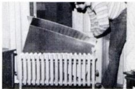
Panel is positioned. A 2-in. clearance is allowed at top and behind radiator.
