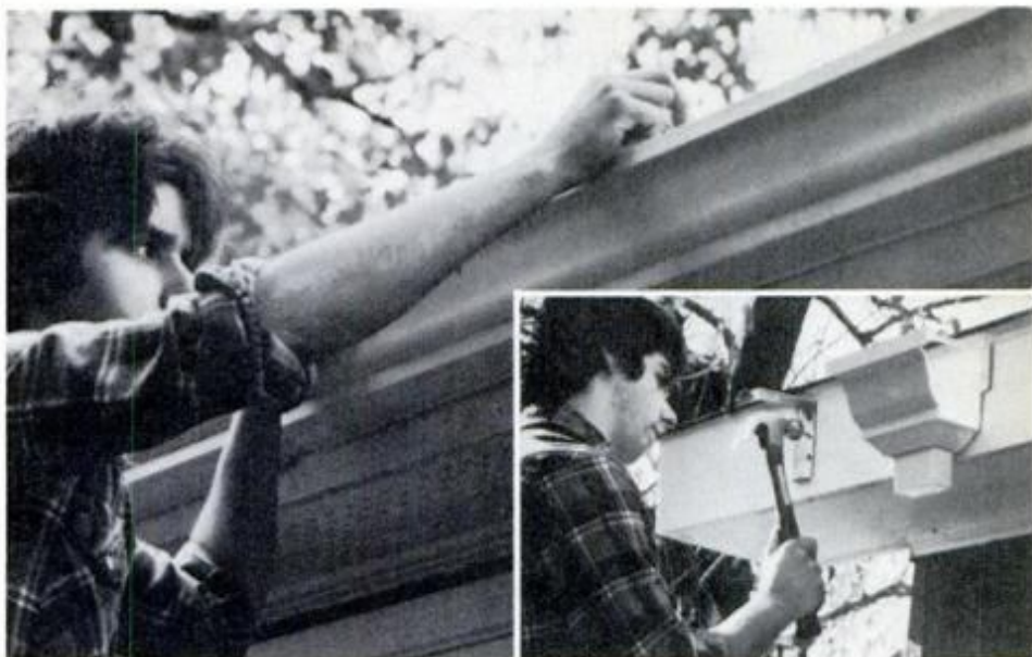
Final touch: Gutter hanger is snapped into gutter lip to complete installation.
