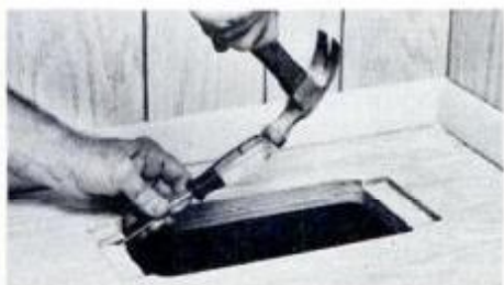
Use a chisel or router to cut the 1/4-in.-deep mortise for the safe's flanges.
