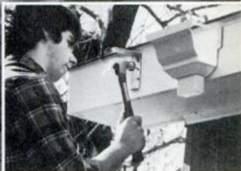
Drop outlet goes up first, then gutter brackets are installed along chalkline.
