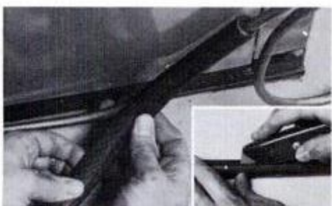
Oil feed line to burner was protected by slipping old garden hose (slit on one side; see inset) over the exposed tubing.
