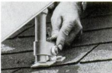
Since roof is pitched 42°, short legs at top bring panels to the desirable 45° angle.
