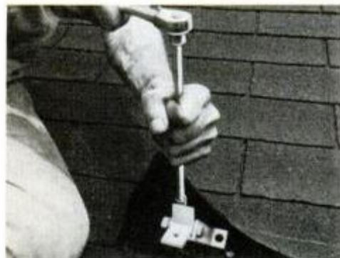
All brackets on the job were installed using lagscrews into rafters, cats or blocking.
