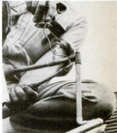
Plumber did some soldering on roof to end the need to carry assembled sections up.
