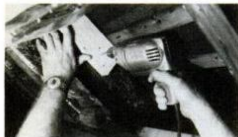
Solid fastening for collector hardware is a must. Here, cat is located and predrilled.
