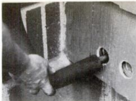
Copper piping for solar fluid was run on the outside of house to avoid a mess inside.
