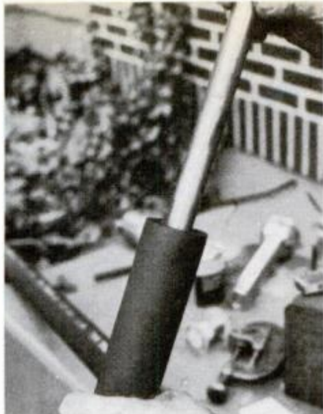
To minimize heat loss as fluid travels, pipe must be wrapped with insulation.
