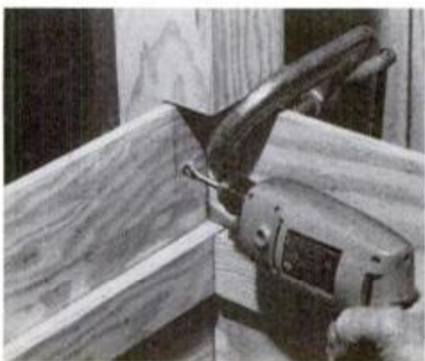
Post should be held securely in place—a C-clamp is being used here—while you bore the pilot holes for the screws.
