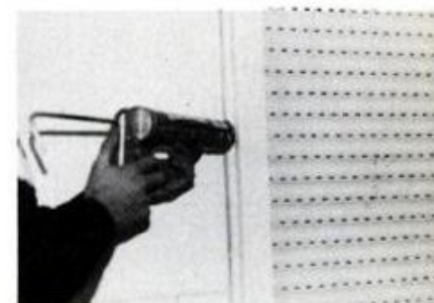
Final step of the installation is caulking the top and both sides of the shutter perimeter in order to seal the unit.
