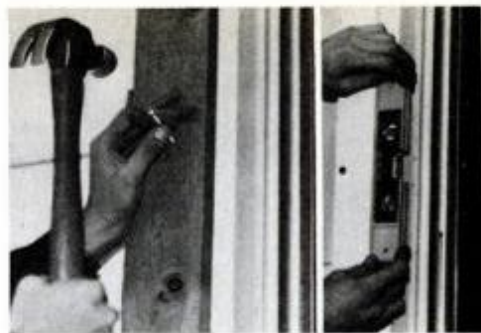
Nail 3/4-in.-thick wood strips at sides and top of door opening (left). Test-position shutter rails on strips, use level to be sure rails are plumb (right). This will insure smooth shutter operation.
