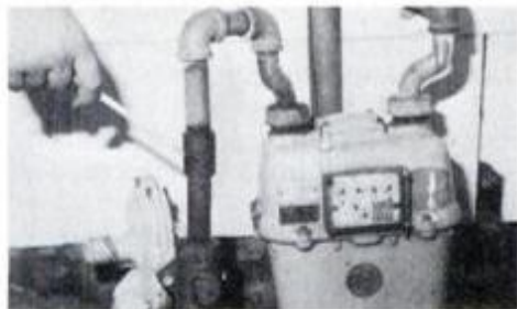
Slipshod gas-meter installation joins galvanized and nongalvanized pipes. Eventually, galvanic action may create leaks.
