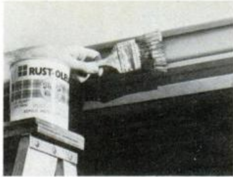
A coat of quality metal primer is a must for a job that will last. Or, use a new water-based primer to speed up the task.
