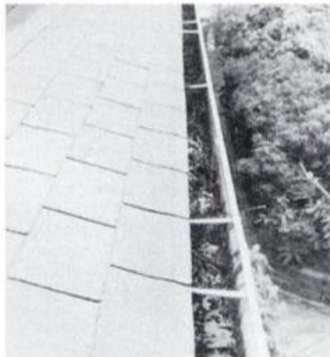
Poorly maintained rain gutter will develop crevice corrosion and soon rot. Gutters should be dry when it's not raining.
