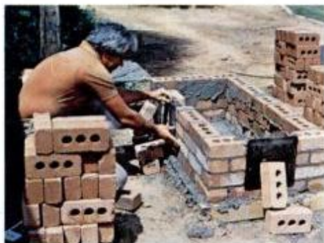
Begin work by laying bricks for the firebox and installing the firebox door.
