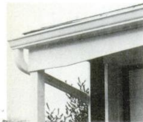
Sanded, primed and topcoated, the old gutter installation now looks like new.
