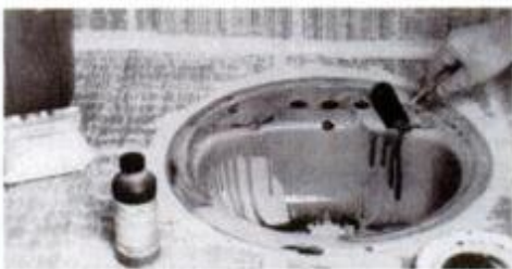
An acid etch removes all of the original glaze to give "tooth" for the finish coat.
