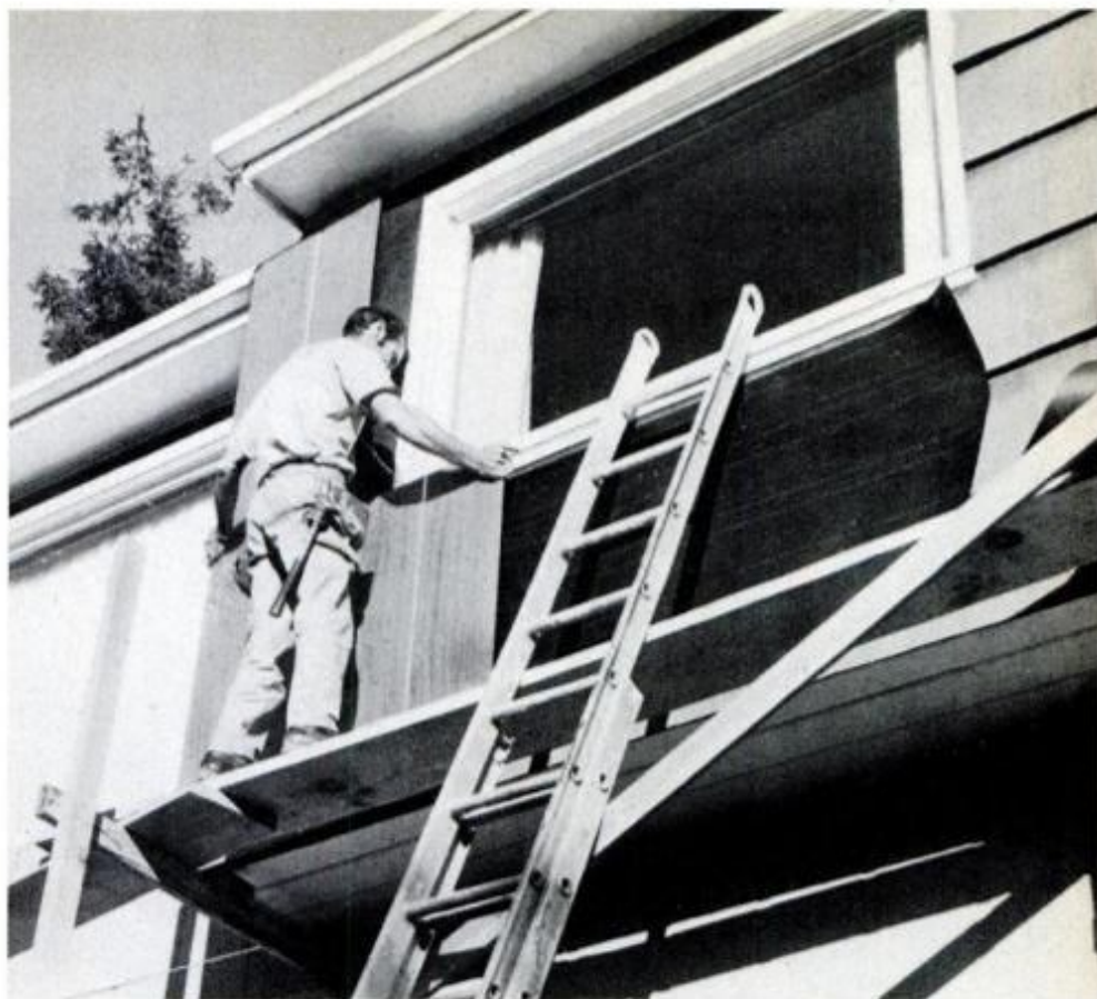
A quality job includes foam-board insulation and attention given to details. Jamb extenders should be used to build out a window frame so it will extend beyond the new siding surface. Inspect at least three jobs by a contractor before hiring him.
