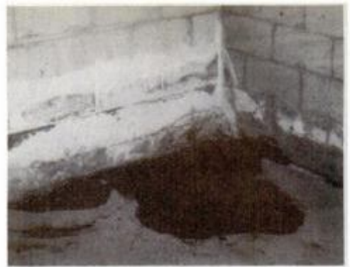
Efflorescence (white chalky substance) stains on walls and floors are telltale signs of water seepage in the basement.
