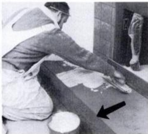
11 Draw line (arrow) where full tiles start. Apply skim coat of mortar.
