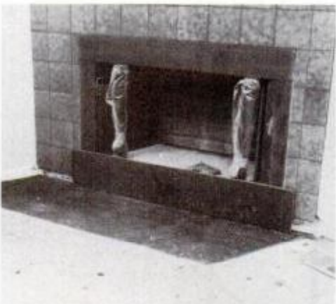
7 Wire lath is nailed to plywood to anchor mortar bed for the raised hearth.
