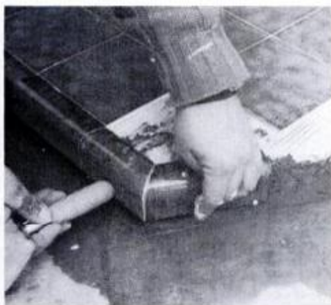
14 Corner tiles must be mitered using a power saw with carbide blade.
