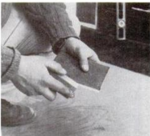
5 Use a carborundum stone to smooth rough spots on cut edge of each tile.
