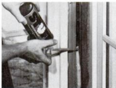
4 Urethane foam from can insulates the crevice around the sliding doors prior to installing paneling on the walls.
