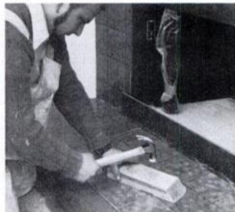
12 Level and seat tiles in mortar by tapping the board with a hammer.
