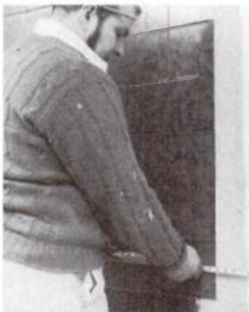
3 Next, measure for the width of border tiles which must be cut.
