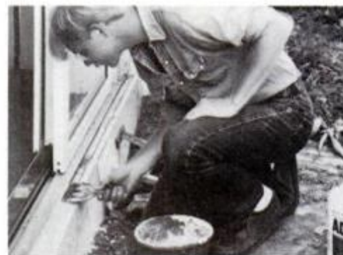
6 To seal cracks and protect exposed surfaces of rigid insulation, apply coat of Thoroseal mixed with Acryl-60.
