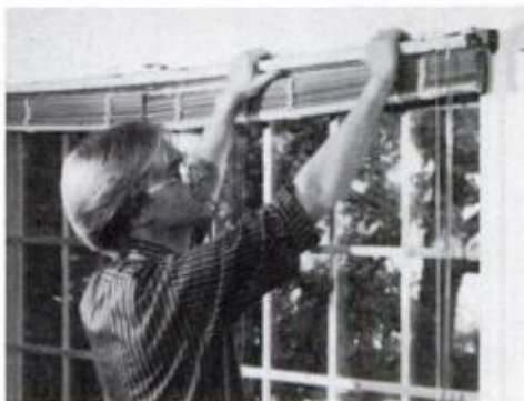
10 Installing blind headrails on face of door casing allows blinds to clear the door pulls without snagging.
