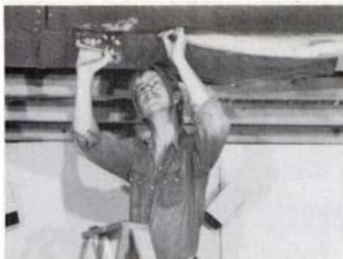
7 Fiberglass batts, Kraft-backed side down, are stapled between ceiling joists following electrical and duct work.
