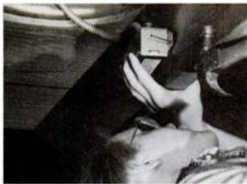
1 Powered roof vent in the attic space exhausts any summer heat buildup and reduces the heat pump cooling load.
