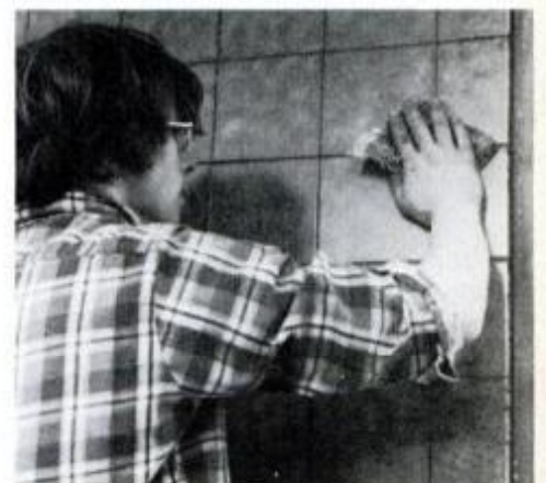
16 When grout starts to set, wipe excess from tile face with sponge.
