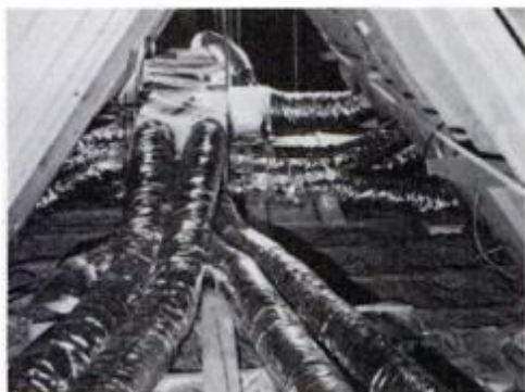
8 Insulated air-handling ducts transfer solar heat to the heat pump and to rooms on the north side of the house.
