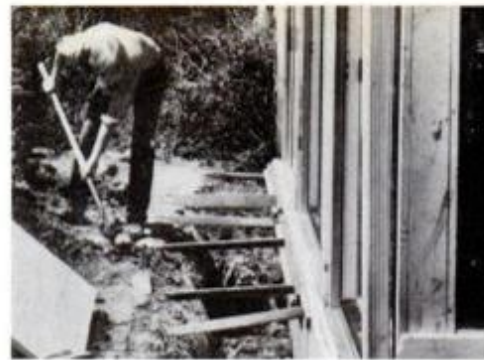
5 Rigid foam insulation around foundation and heat sink (existing slab) reduces heat loss at building perimeter.
