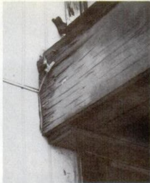
Rotten fascia is caused by lack of caulking at the joint and/or no drip edge or shingle overhang along the eaves.
