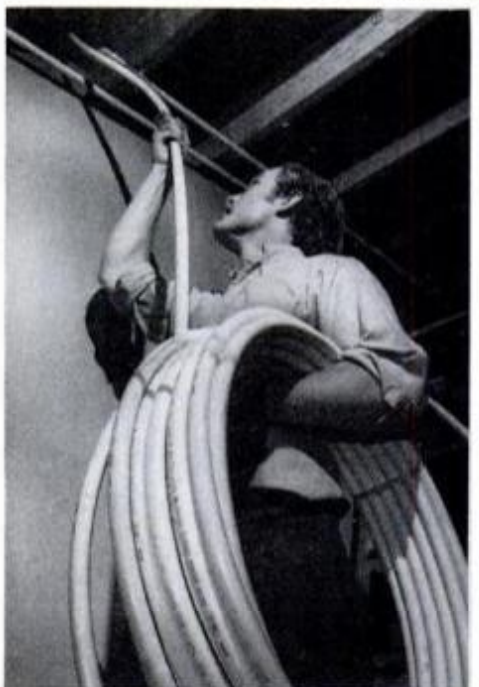
When piping must be fitted behind walls or fished through openings, use flexible PB to save your time and effort.
