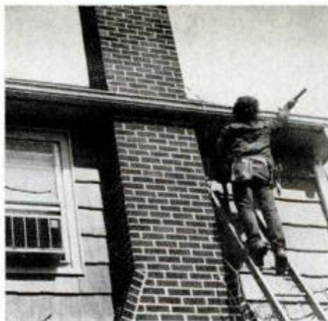
Patch job started with removal of the existing gutter and fascia board behind.
