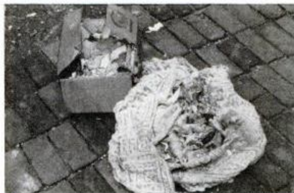
Using a bedspread and other materials found in attic, squirrels fashioned a super-comfortable nest (above). Wiring on fan stored in attic (right) was chewed and destroyed by squirrels.
