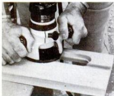
5 Cut rabbet around the back of ball-return opening to reduce wall thickness and make reaching balls easier.
