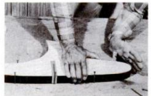
As you bend steel runner edge to shape, lock it in place with more nails.
