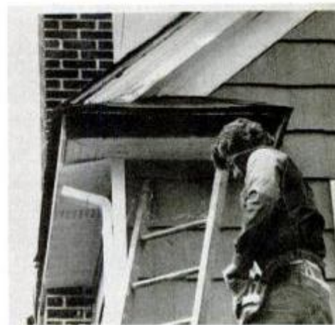
To prevent future entries, soffit and fascia are both enclosed with metal.
