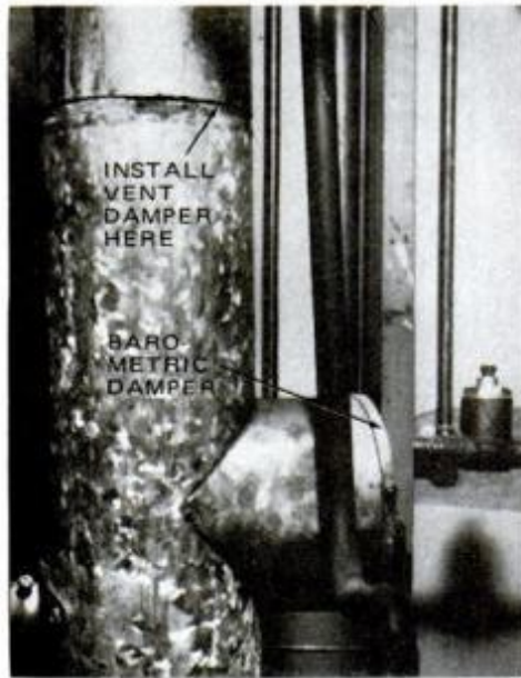
Photo of existing setup shows where automatic vent damper should be installed, between chimney and barometric damper.
