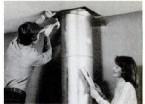
Run pipe through ceiling and roof and fasten firestop to top of ceiling header.
