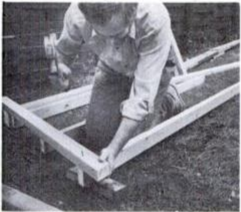
Cut waste from tops of studs and assemble with 16d common nails before raising.
