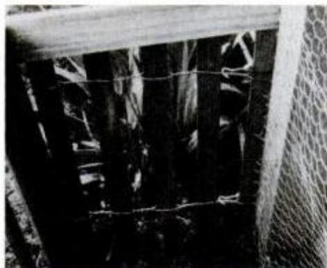
Top rails of 1x4 connect the garden fence posts to the existing yard fence.
