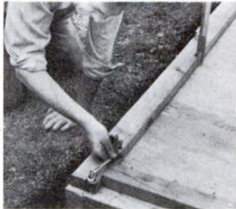
Set electrical conduit and anchor bolts in concrete; fasten sills with bolts.
