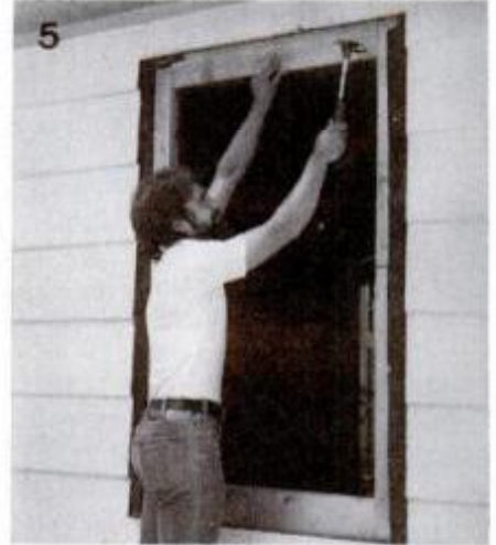
5 Sheath new framing flush with existing sheathing. Rough opening is now ready to accept the new window unit.
