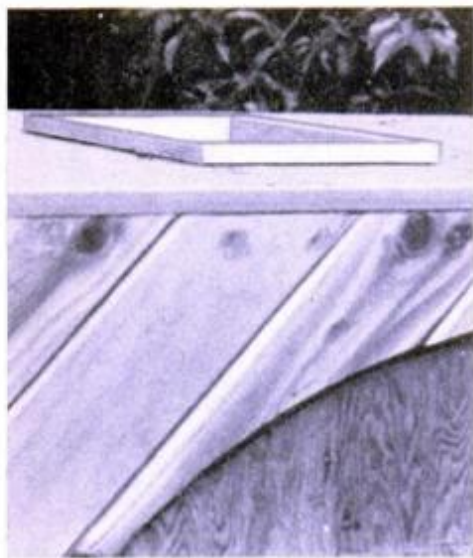
Hatch opening is cut between two rafters, trimmed with cedar and then fitted with sheet-acrylic lid. Note: Roof access may not be safe for very young children.
