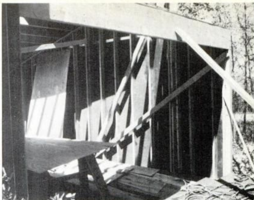
Wall framing is held plumb with temporary diagonal bracing until framing is in and walls covered both sides.
