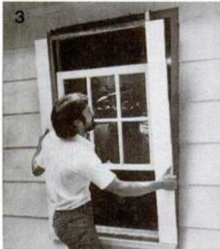
3 Lift out the window from outside after using wrecking bar (if needed) to finish popping old unit from opening.
