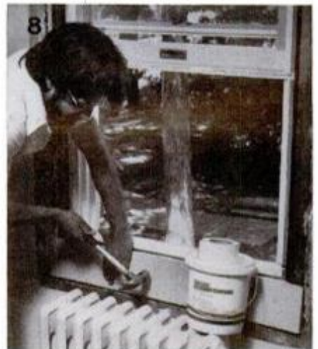
8 Nail drywall patches over areas which interior trim will not cover. Tape and spackle all exposed joints.
