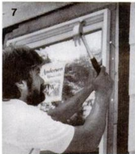
7 Nail window to wall. Fin-type window, shown, has vinyl flange for nailing—others are nailed through casement.
