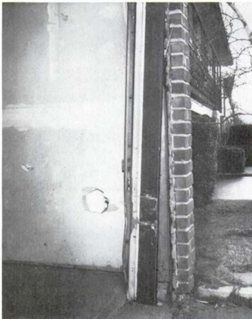
Off-target car approach resulted in jamb being shoved to rear. Track was knocked out of alignment, brick veneer separated from sheathing.
