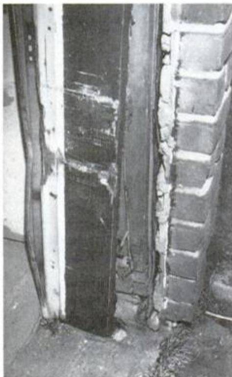
1 Twisted steel track makes it difficult—often impossible—to close door.
