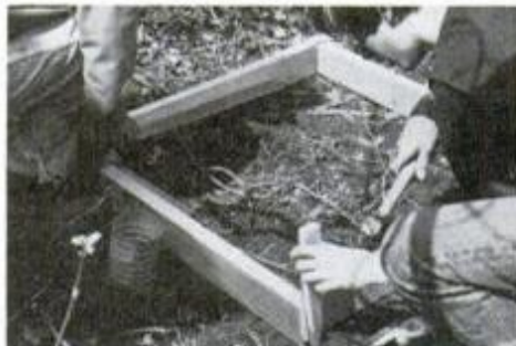
1. Generator sits on a 30x30-in. concrete pad. Use 2x4s, stakes for forming.
