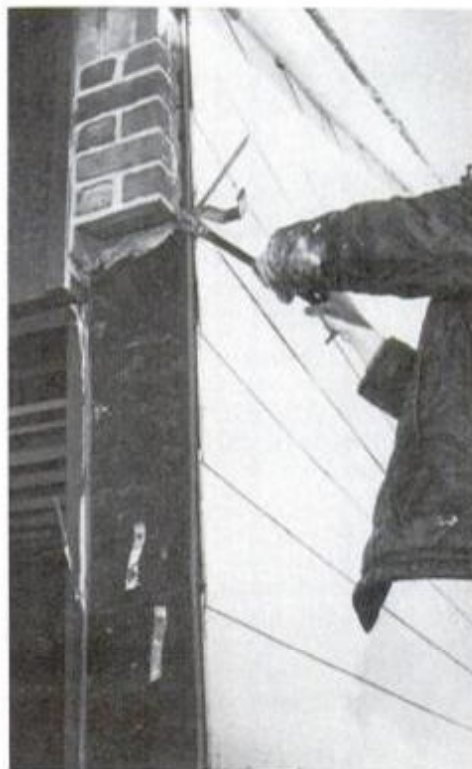
2 Damaged brick is removed by wrecking bar. Safety glasses are a must.
