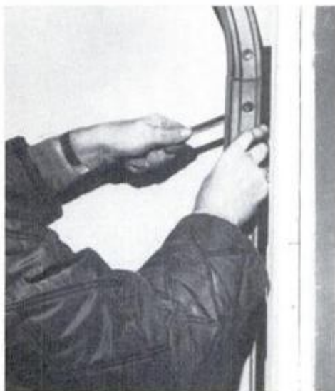
8 Finally track is returned to original position and refastened to angle iron.
