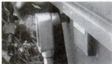
9. Branch circuit from house enters the generator housing through a conduit.
