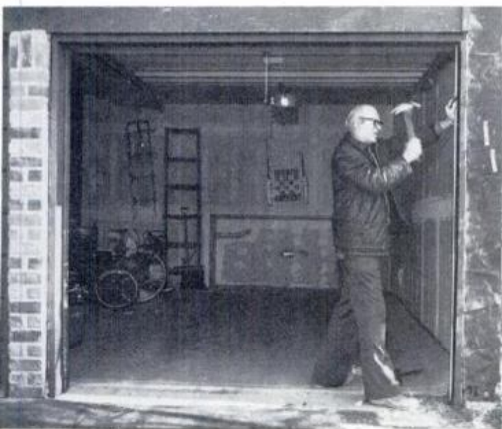
10 Pull overhead door down, test fit. Finish renailing jamb to framing; set all nails and fill with putty.
