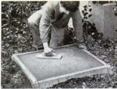
5. Next, surface is floated to fill voids left by straightedge and embed aggregate.
