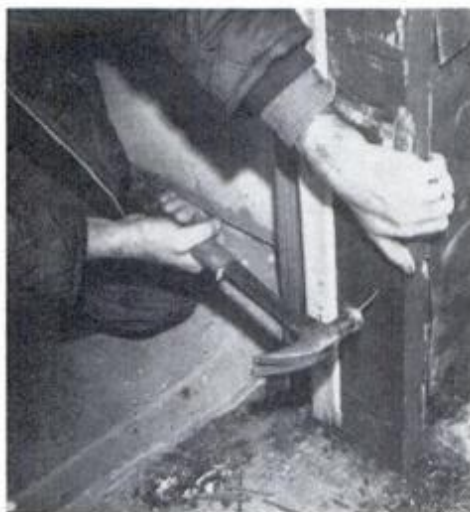
5 Realigned jamb is then checked for plumb and nailed to the framing.
