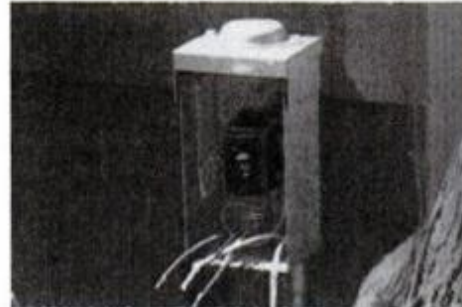
8. Box for generator main circuit breaker, mounted on house, takes 30-amp. breaker.
