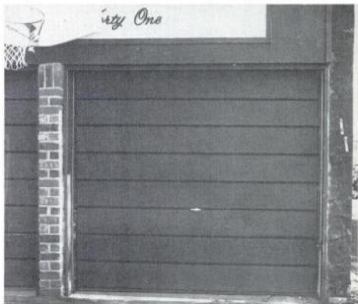
11 Replacing the brick veneer is still to come—but at least owner can now close and lock the garage door.
