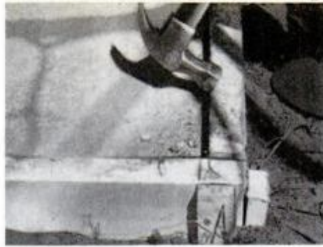
6. Let concrete cure for 24 hours, then "crack" forms by tapping with a hammer.
