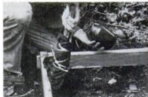
2. Tie rags on a stick to oil form inside to keep concrete from sticking.
