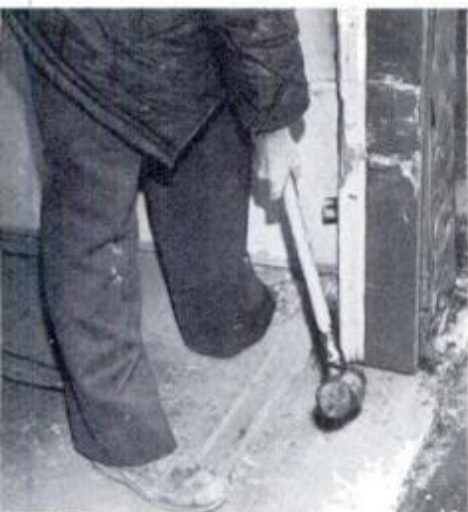
4 Mallet is used to gently ease salvageable door jamb back into position.
