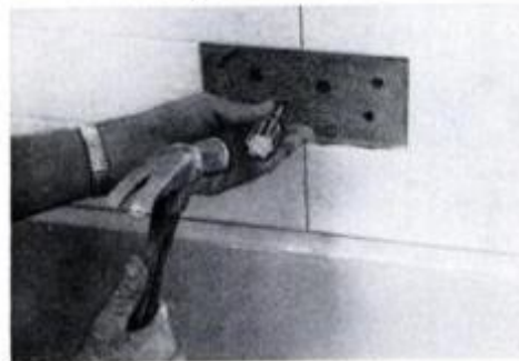
19 To install soap dish, punch holes in board with a hammer, screwdriver.
