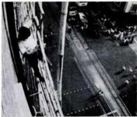
Hong Kong scaffolders use no planks. They cling to a bamboo jungle gym.
