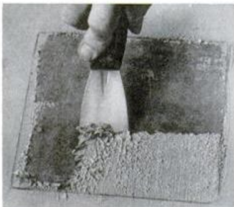
Thoroughly strip all paint from patch with a scraper, exposing bare concrete.
