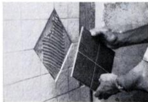
18 After pre-cut sheets of tile are in place, insert the diamond section.
