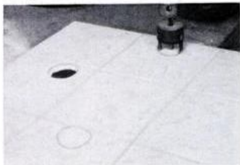
15 Drill pipe holes in tile. This one is Redi-Set pregrouted sheet tile.
