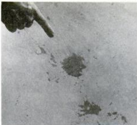
Pick a bare spot where blistering has occurred and mark off patch for removal.
