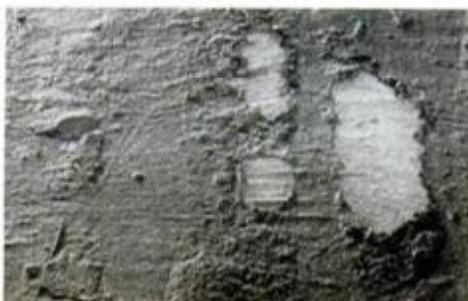
BLISTERING AND PEELING. Diseased paint lifts off surface and crumbles away, due to moisture in concrete that dissolves alkali, carries it under paint.
