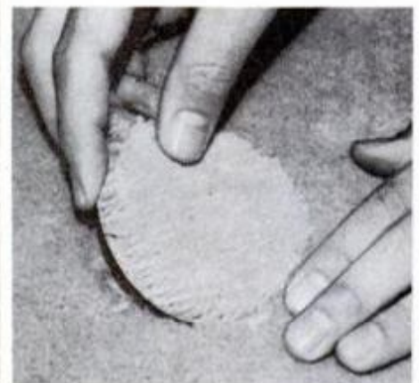
Press the carpet round down firmly to adhere. It will accurately plug the hole.
