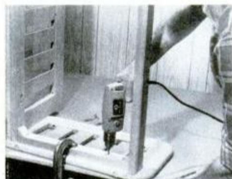
11 Clamp seat frame to side and back while you bore screw pilot holes.
