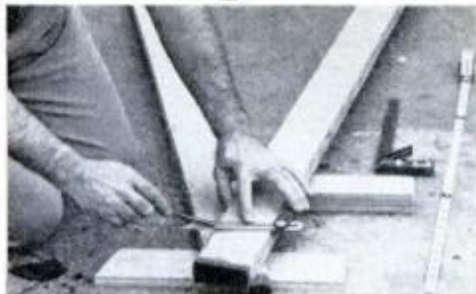
12 Lay frame members on floor. Mark for miter cuts. Set T-bevel for 105°.
