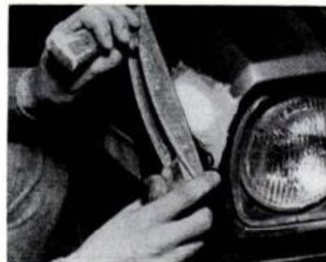
Shape the hardened filler as close to the original contours of the body as possible.
