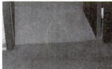
7. The end result is a smooth seam that separates rooms having different carpets.
