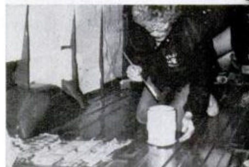
Holes for floor screws could start rust, so author cemented in Ensolite, plywood.
