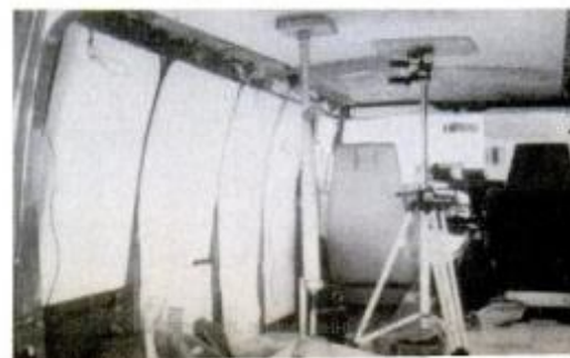
Extra hands help for bowing ceiling into place. Here are jack, bat and tripod.
