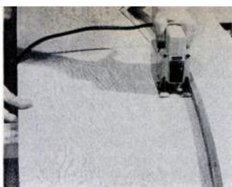
Long curves can be cut with flexible guide-strip tacked in an offset position.
