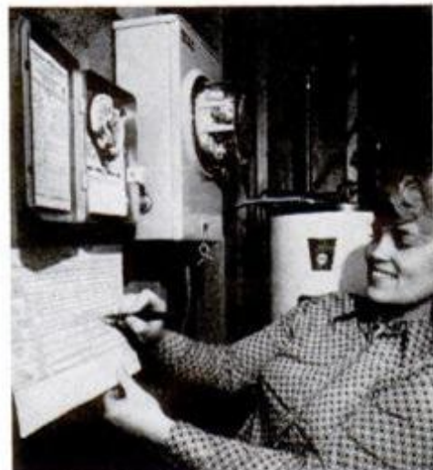
Wisconsin transponders are in box below customer's meter. Water-heater remote switch is located beside electric meter.
