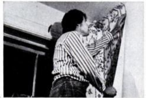
6 Unfold top part only, position it near the ceiling with 3 in. overhang. Line the edge with a plumb line and smooth it.
