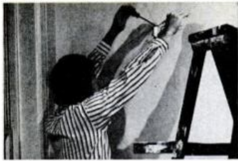
1 Remove plant hangers, switch plates, hardware. Turn off electricity at fuse box and pull fixtures away from the wall.
