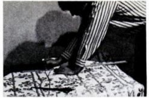
3 Measure ceiling height. Allow 3 in. extra at the top and bottom. Cut a strip. Match the pattern and cut two more strips.
