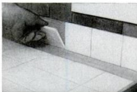
8 Tiles on backsplash exceed its height by ¼-in. to allow for edge tiles.
