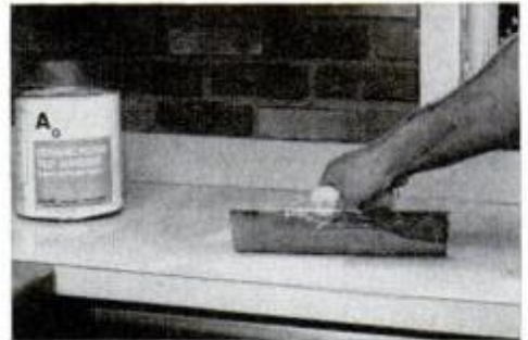
3 Apply suitable adhesive (see text) and spread it evenly with a notched trowel.
