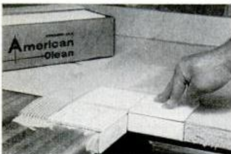
4 Install tile along edge with ¼-in. overhang so it will top off edge tiles.
