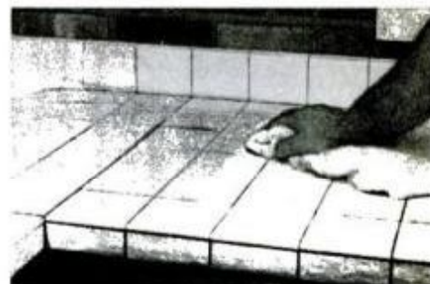
18 Polish tile with a clean, dry cloth, then reinstall sink and job is done.
