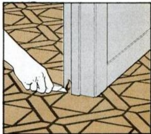
With sharp utility knife at a 45° angle, carefully trim off the excess flooring.
