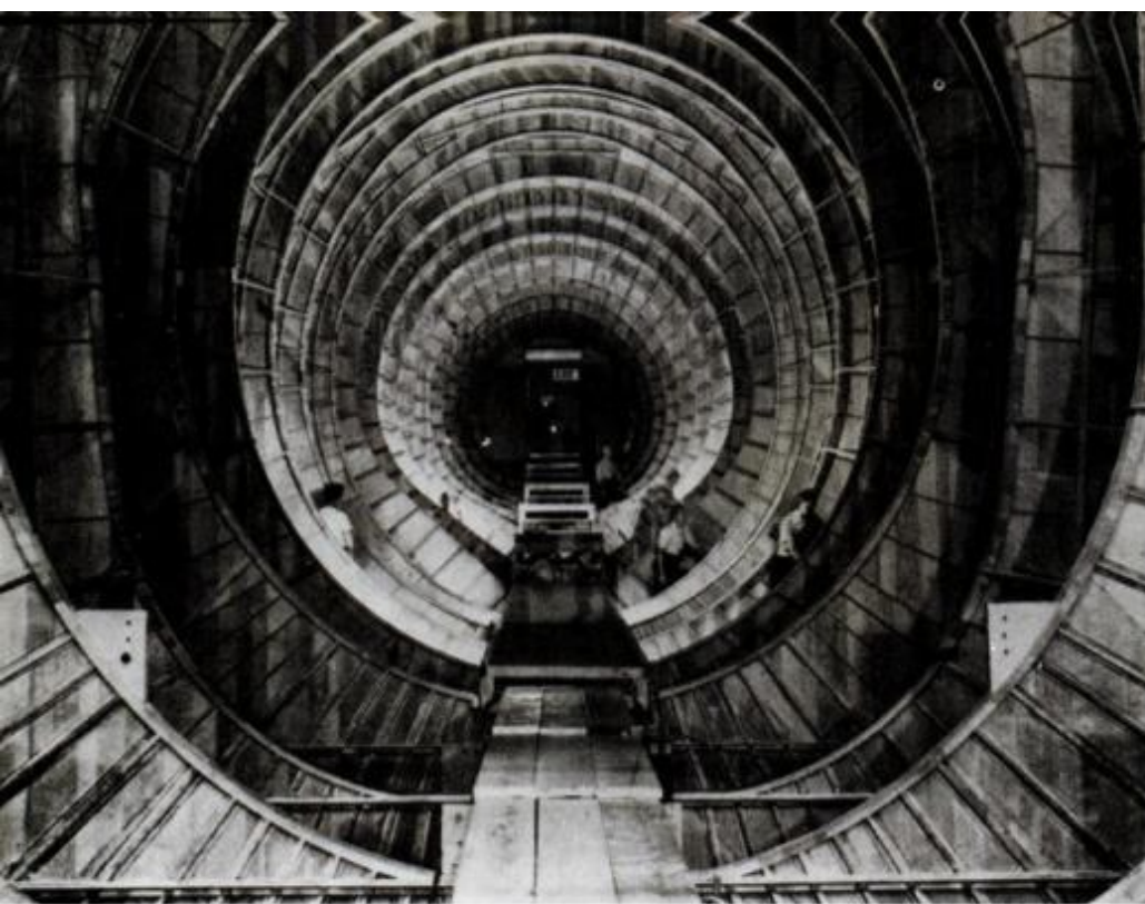
H-4 interior under construction, looking aft (above). Vast deck, when completed, was designed to support 60-ton tanks and armored vehicles. Hull is 25 feet wide by 30 feet high.
