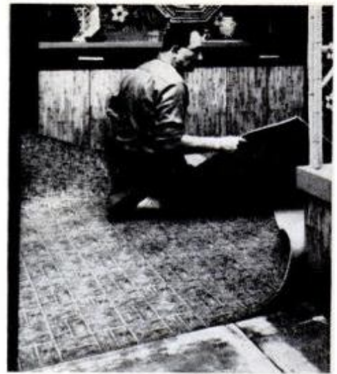
The first step to install seamless flooring is to position it in the room.
