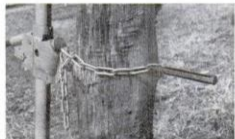
Chisel and chain—with links hung on the jack's lifting hook—connect post to jack.
