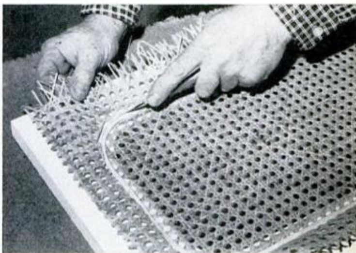
Trim off the excess with a razor knife when glue in the groove has dried and the cane has dried taut. A liberal allowance of excess cane— 1\frac{1}{2} -in. minimum—makes the installation easier.
