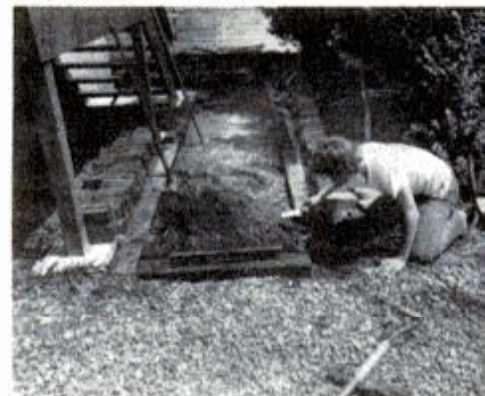
The ground is excavated and the railroad ties are then leveled in position along the perimeter of the excavated area.
