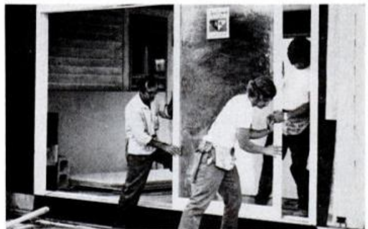
Stationary door panel is installed first. Predrilled holes for fastening of brackets assure proper alignment with the frame.
