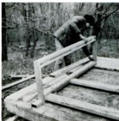
Make up the door frame on the deck. Doubled 2x4s at each corner are tied together with doubled plates and 2x6s.
