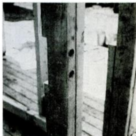
The bench support 2x6 across the door front is notched into the studs and lag-bolted through the end of the stud.
