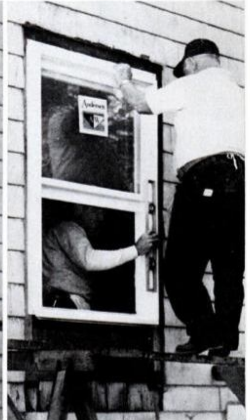
Add sheathing over new framing, cover with tarpaper and set in the window.
