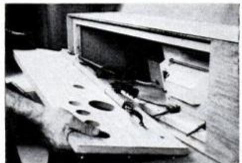
Mount a 25 1/4 in. section of Wiremold multi-outlet to access panel and run power cord from Wiremold cordset out back.
