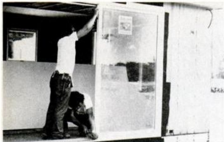
Metal brackets are screwed to the door and frame at the head and the sill in order to lock the stationary panel in place.
