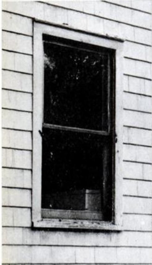
Windows do eventually wear out. Rotting sills or warped sash may be beyond repair.
