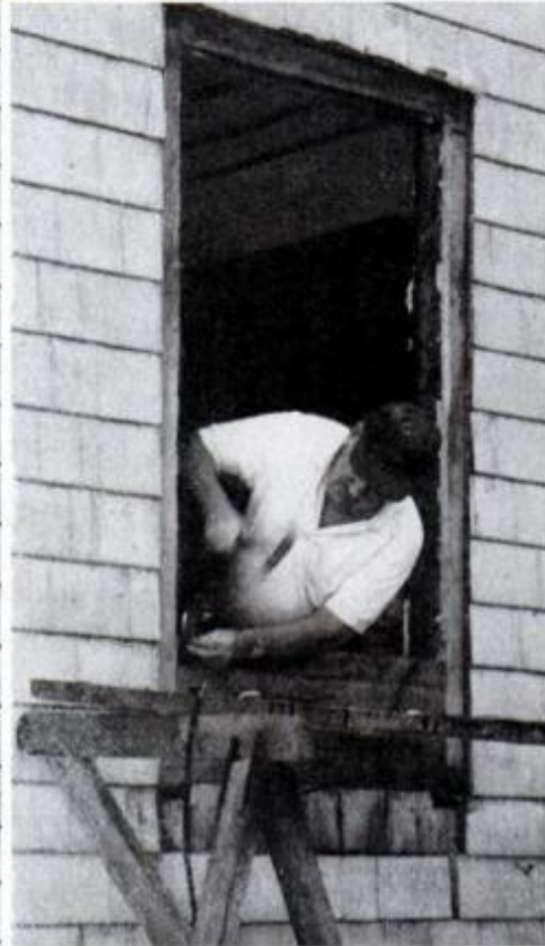
Remove window , add filler studs and sill to fit new unit. Siding stays intact.
