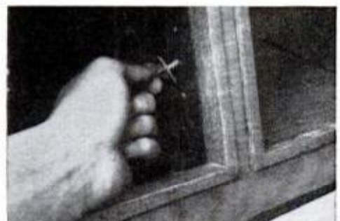
Drill holes front and rear in both shelf dividers for the shelf support clips. Shelves are 1/4-in. veneered plywood.
