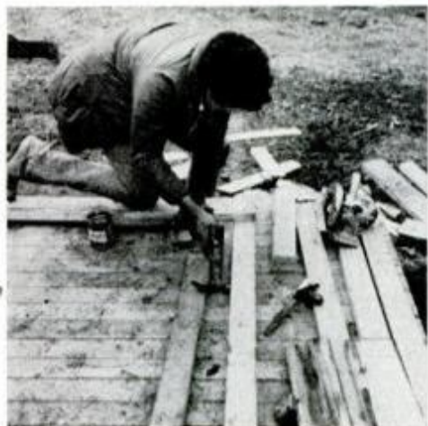
Total door height (including the casters) should be approximately 3 in. less than the shed for the drip edge clearance.
