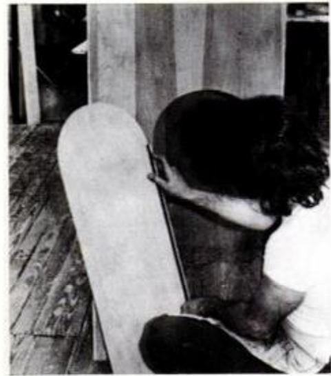
Stage-door hinge is placed in a 1/8-in. recess sawed out of the door. A 1x1-in. wood support strip will be attached later.
