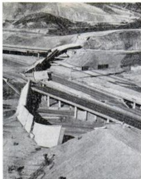
Quakes cause key supports to give way.
