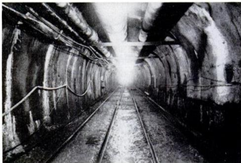
Pilot tunnel, nearly complete, shows two rail tracks, complex array of power cables and ventilation ducts. But appearance is crude compared to how finished tunnel will look.
