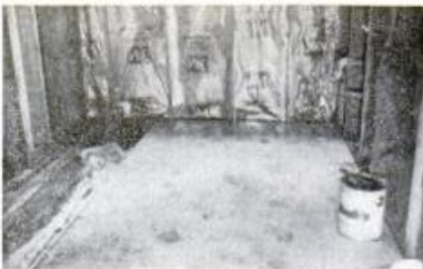
Resurfacing. A new 5/8-in. A-C exterior-grade plywood subfloor provides a durable and solid surface for the ceramic tile.
