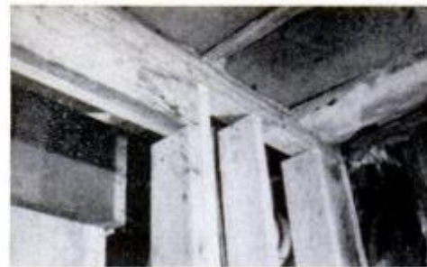
More strength. The wall-hung toilet is supported by a steel hanger that must be bolted through two new 2x6 studs.
