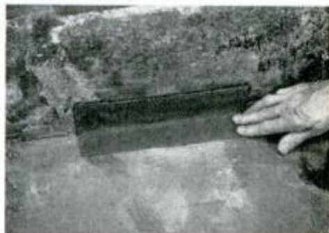
Rok-Rap is used to patch a basement crack where water was seeping in.
