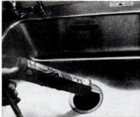
A thin silicon bead inside the flange on the drain basket will make a leakproof seal when flange is tightened down.
