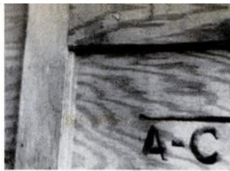
3. Reinforcing. Added 2-in.-wide plywood strips screwed to the 3/4-in. counter provide backing for the laminate edge.
