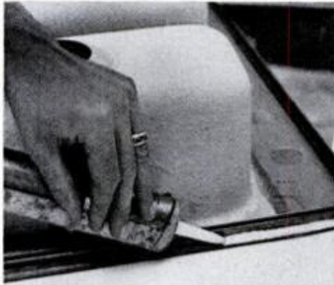
6. Watertight. Use a clear silicon or white butyl bead along the flange. These materials won't dry out or crack.
